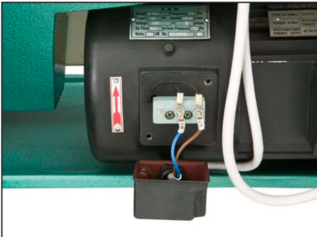
Figure 113. Left motor junction box.
